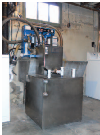
Figure 6. Example of a standard Hg Containment unit .
